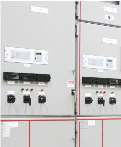
REA relay provides high speed arc flash detection and protection for personnel and equipment.
